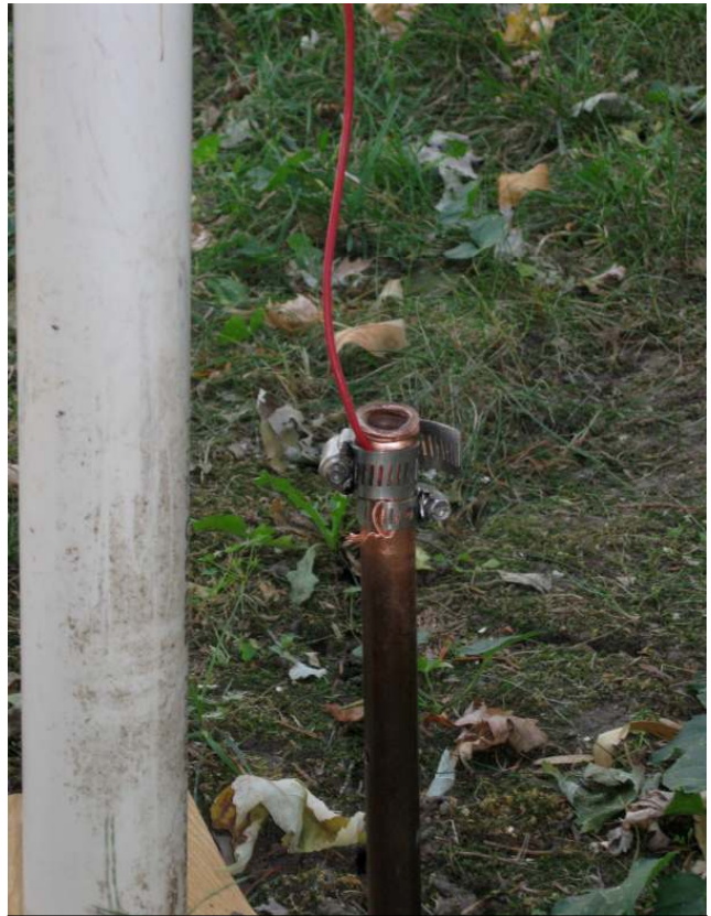
Close-Up Of Ground Rod + Wire From Feeder
